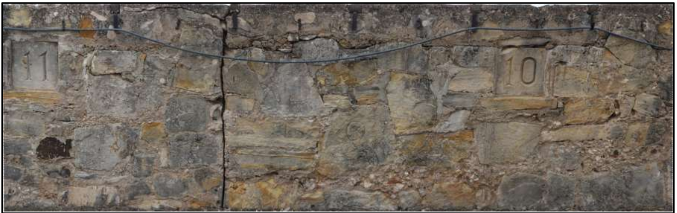
Figure 9 – Stitched panorama covering the range wall from between Stations 10 (right) and 11 (left).
